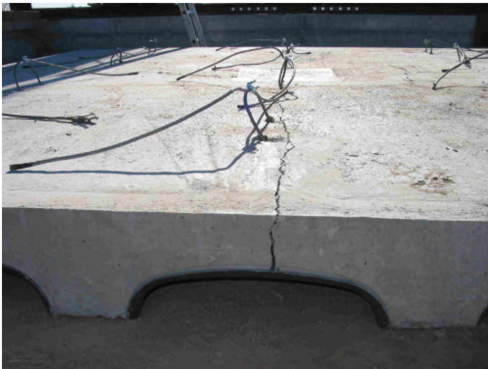
Fig. D.12 Crack line detail on the concrete test n°1
