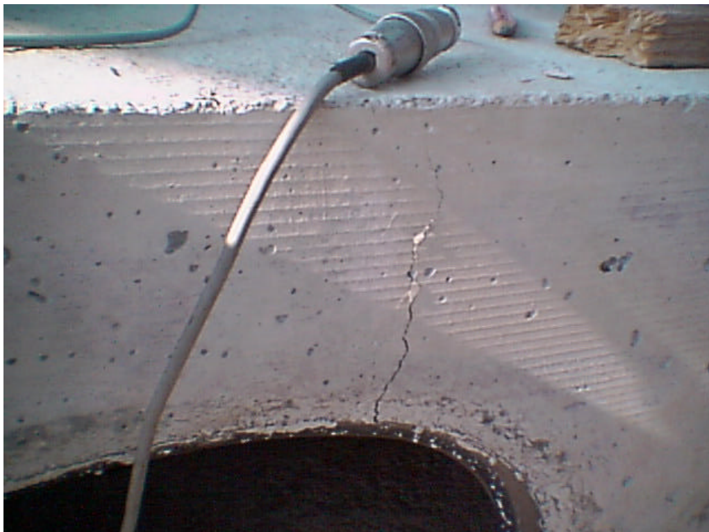
Fig. D.18 Crack line detail on the concrete test n°6
