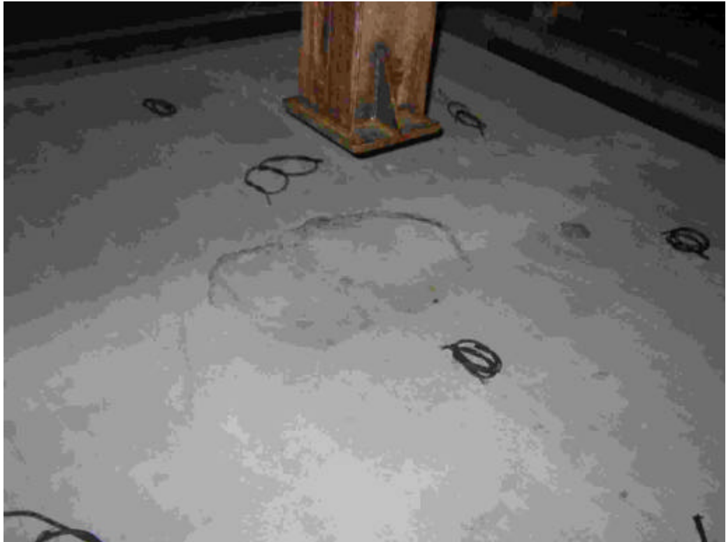
Fig. D.25 Punching Crack on the concrete test n°12
