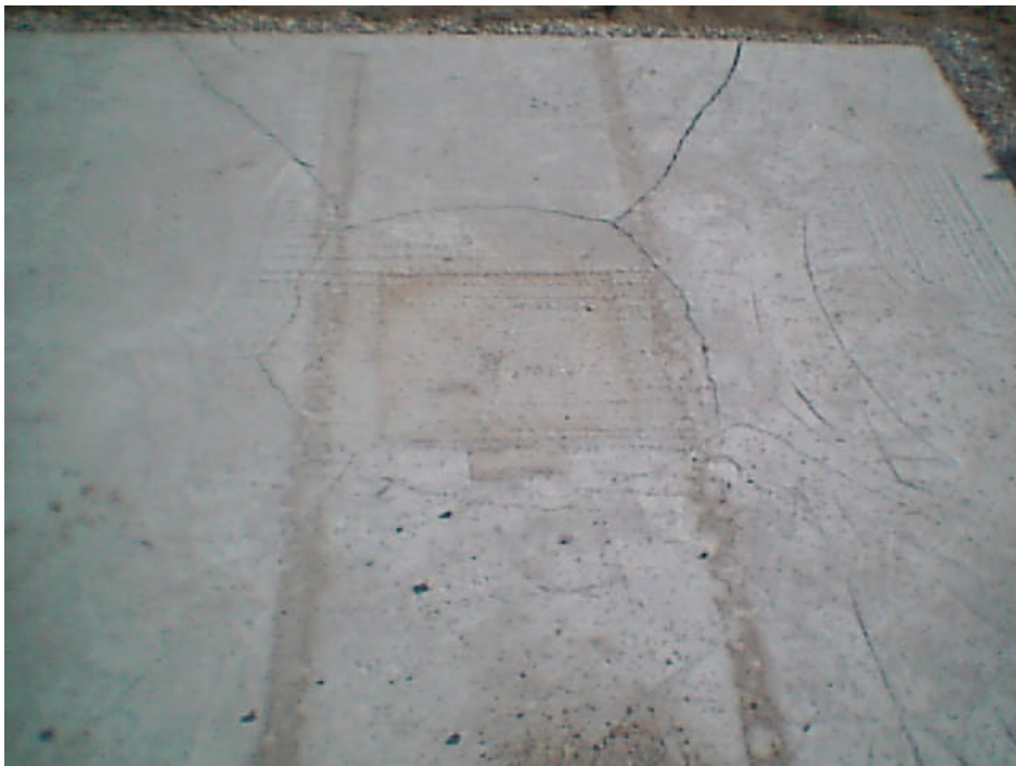
Fig. D.32 Punching Crack on the concrete slab
