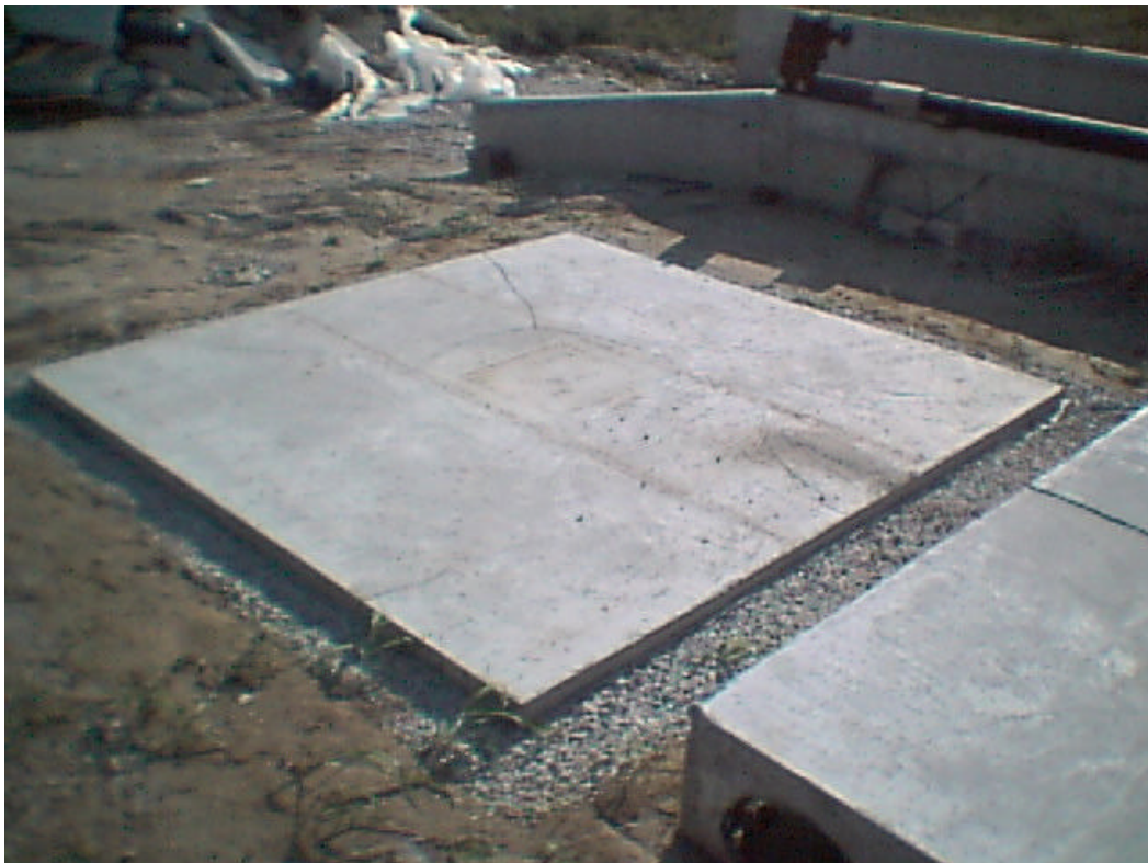
Fig. D.28 Crack line on the concrete slab
