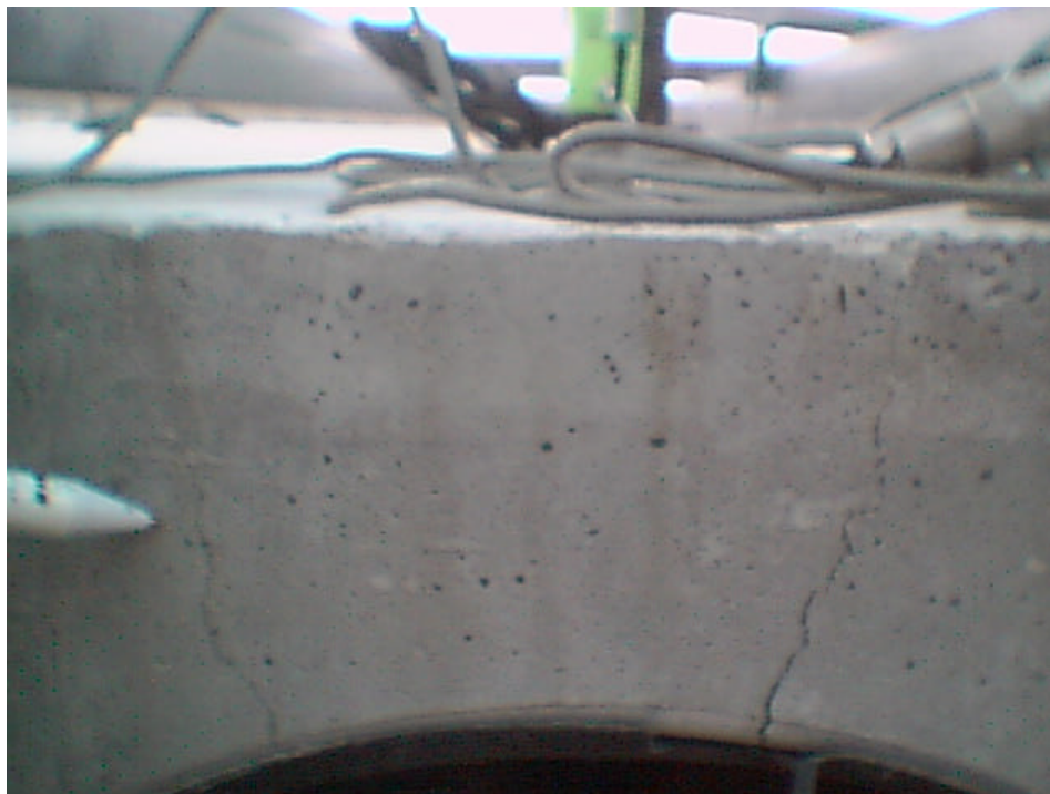
Fig. D.20 Crack line detail on the concrete test n°7
